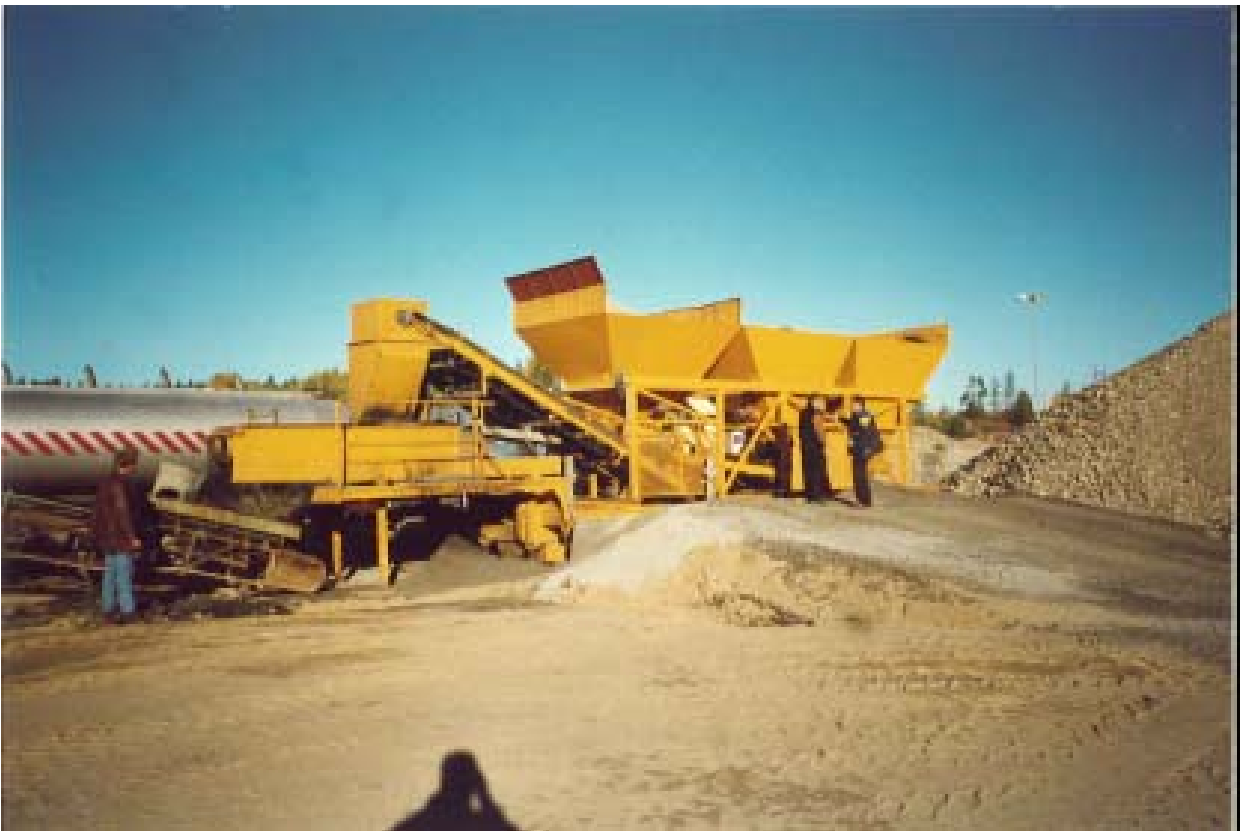
Figure 1. Cold mixing plant used for mixing the crumb rubber with 15 – 25%(weight) bitumen emulsion (the percent figures refer to the net weight of dry bitumen added the crumb rubber) . About two tons of rubber granulate 0-0.5 mm and 0.5-1 mm was pre-treated/impregnated using the plant shown above.
