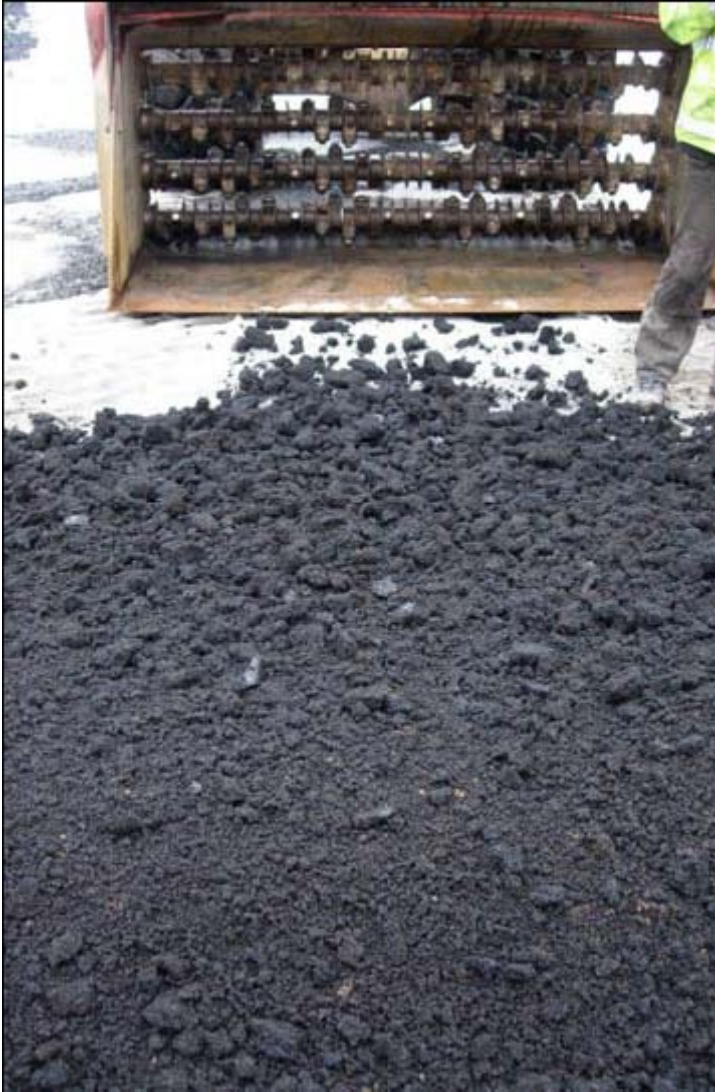
Figure 4. Disintegration of the bitumen impregnated/pre-treated crumb rubber to powder ready to be added in the plant mixer.
